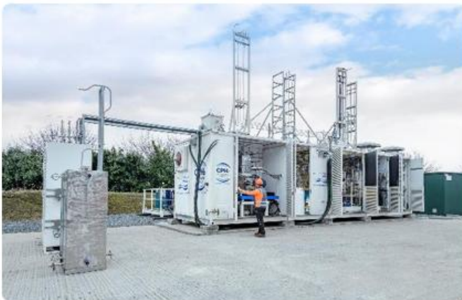
CPH2 MFE 110 at NIW WWTP Site
